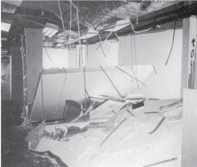
Figure 60 - Partitions and ceilings toppled onto office spaces during the 1994 Northridge Earthquake.
