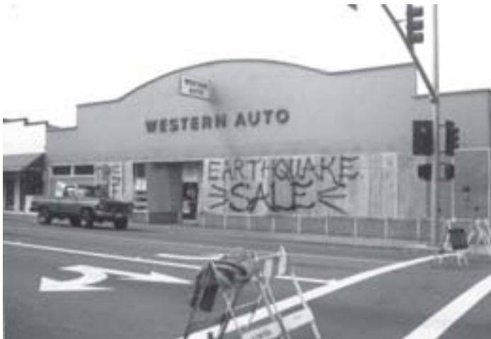
Figure 55 —The front window of this Fortuna auto parts store broke in the 1992 Cape Mendocino earthquake.
